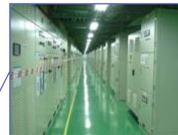
108MVA AVC Wuxi. China
